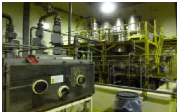
Gambar 4.4 Unit Chemical Treatment
