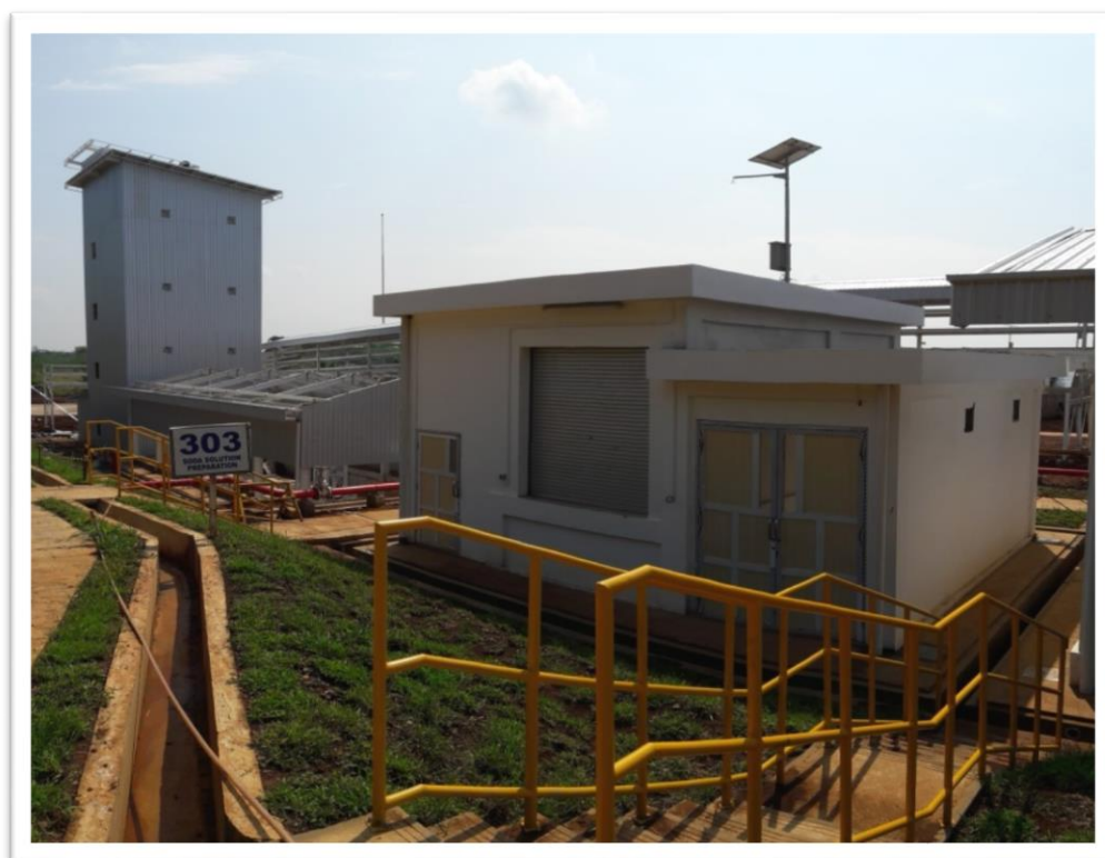
Foto Glycerine Storage and Soda Solution Preparation
