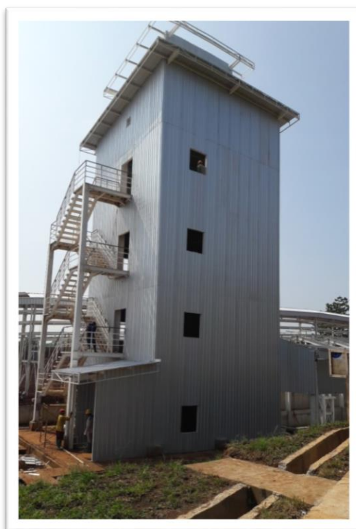
Foto Spent Acid Post-Separator
