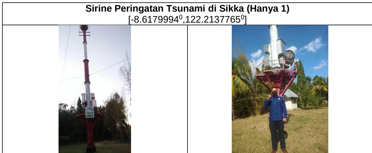
Gambar. 4.59 Sirine Evakuasi Peringatan Tsunami
